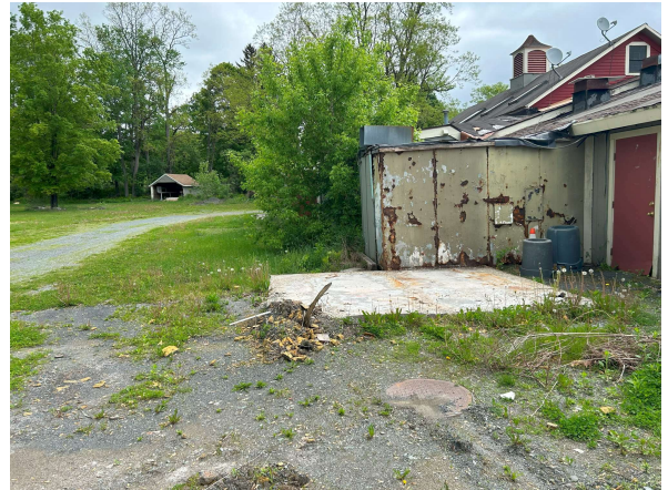
Photo #10 Manhole cover and concrete slab located on the rear side of the site building
