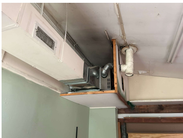
Photo #17 Heating unit located within the site building
