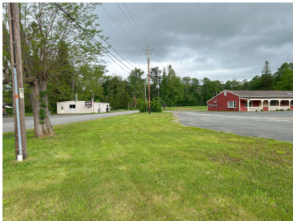
Photo #3 Southwest corner of the site where pole-mounted transformers are located
