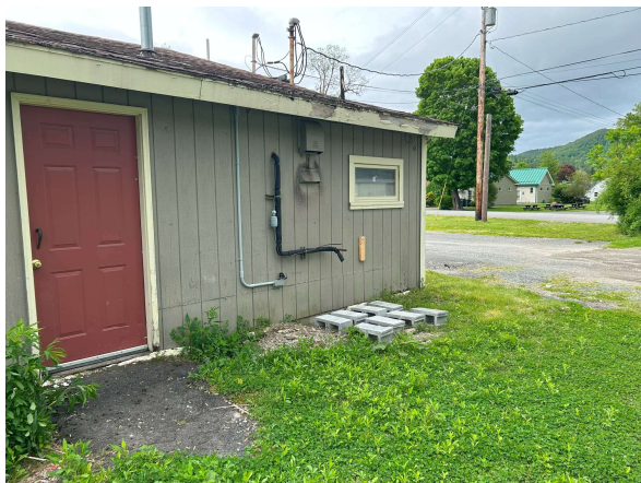
Photo #11 Formerly utilized propane connection on the rear side of the site building
