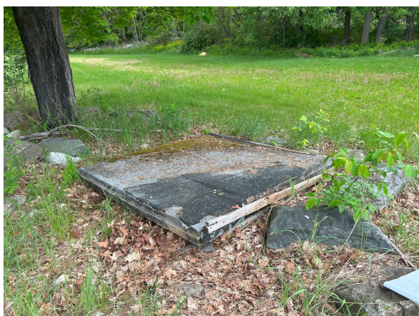
Photo #5 Potable water well vault (cover)
