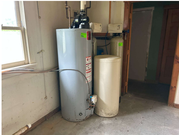
Photo #13 Water tank and water filtration system
