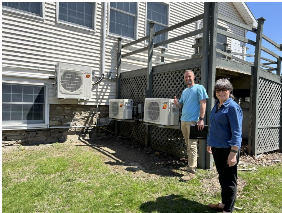
Canaan Town Supervisor Brenda Adams and Paul Fontaine from Ridgeline Heating and Cooling with Canaan’s heat pumps.
