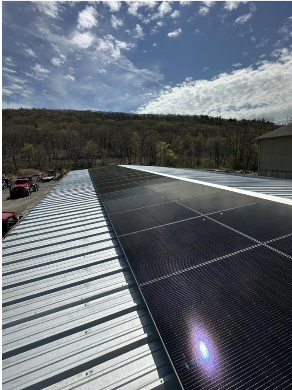
Solar array on Canaan's Highway Garage.
