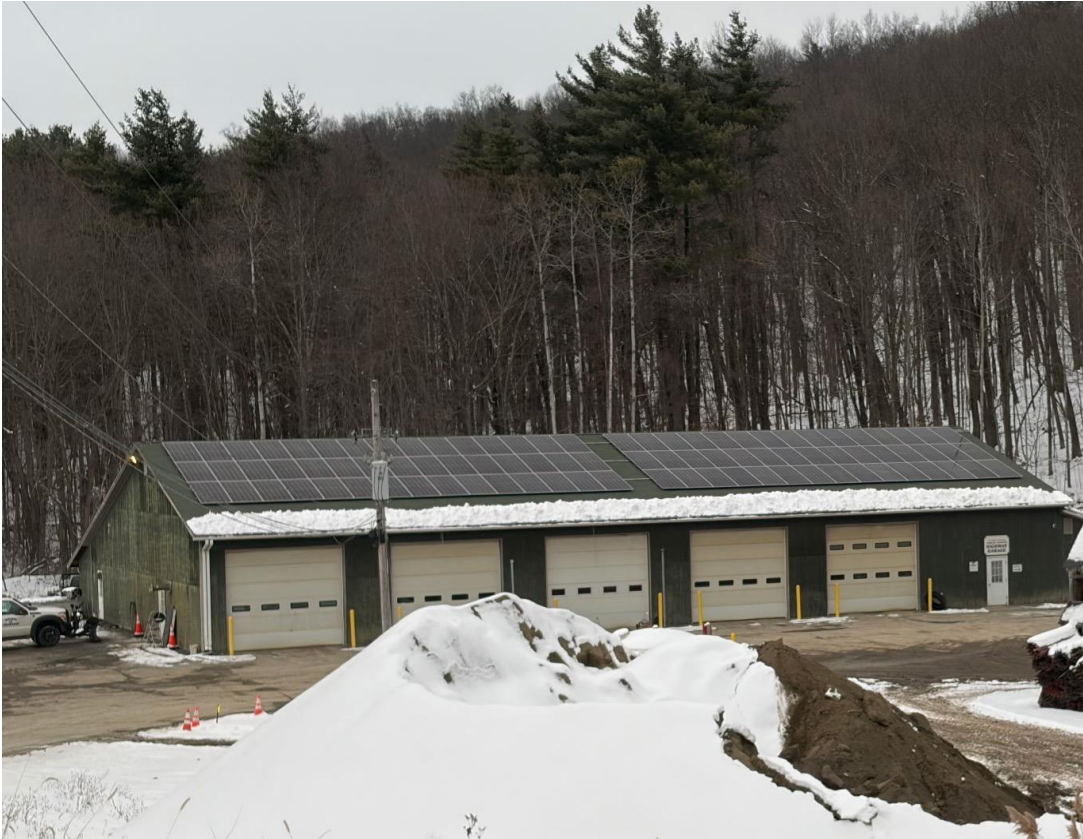
Solar array at Chatham Highway Garage
